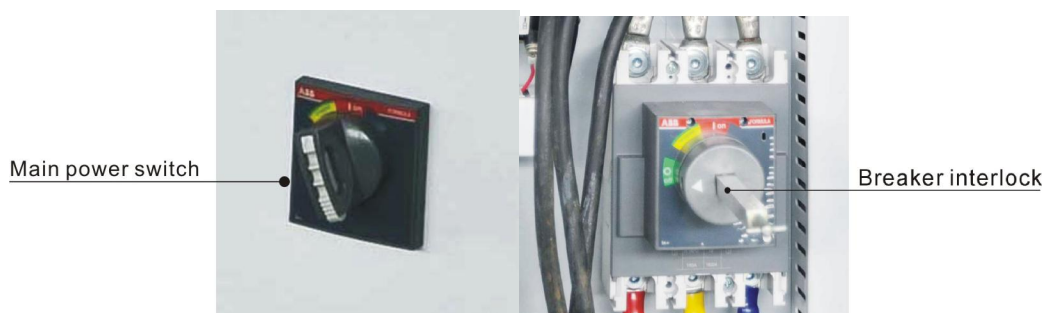
Picture 4-5: Main Power Switch
