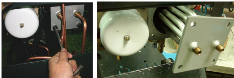
Picture 6-9: Cooling Pipes 2
