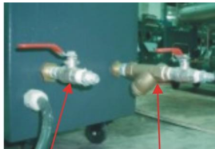
Cooling water outlet Cooling water inlet
