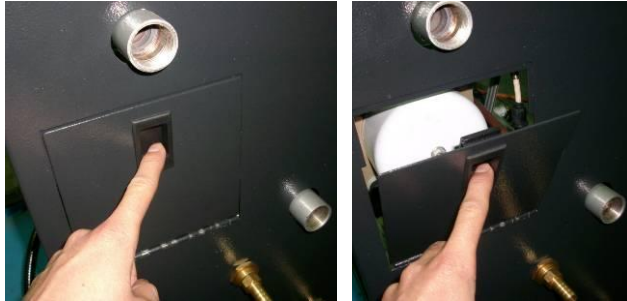
Picture 6-6: Pipe Heater 1
