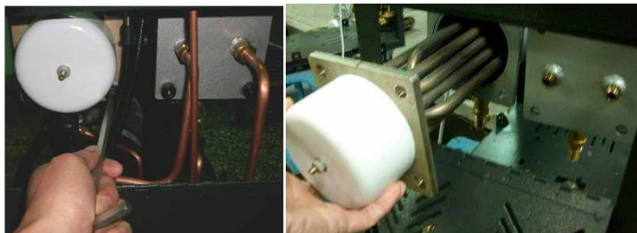
Picture 6-7: Pipe Heater 2
