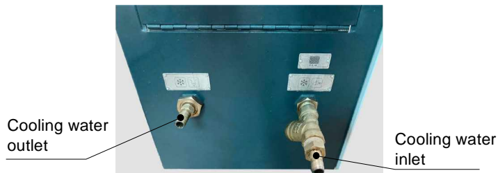
Picture 3-2: Pipe Connection
