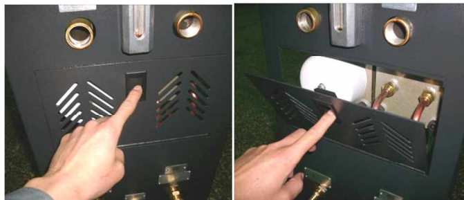
Picture 6-6: Pipe Heater 1
