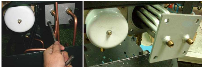
Picture 6-9: Cooling Pipes 2
