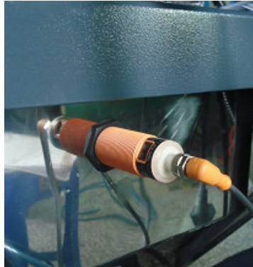
Picture 4-29: Level Switch on storage Tank
