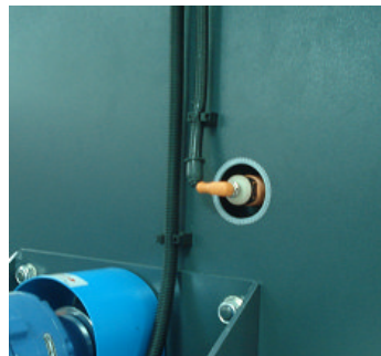
Picture 4-28: Level Switch on Mixing Tank
