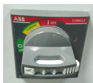
Picture 2-2: Main Power Switch
