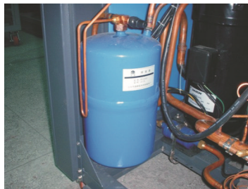
Picture 2-8: Fluid Reservoir
