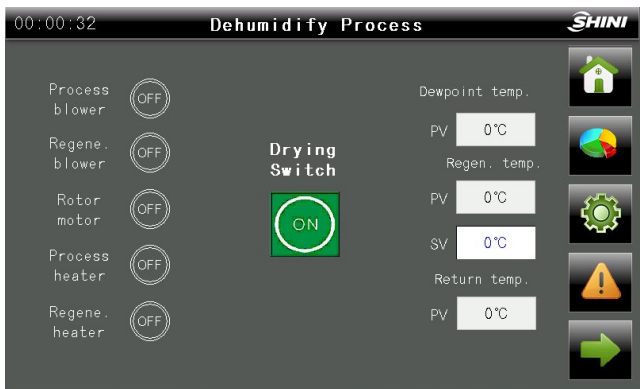
Picture 4-12: Dehumidify Process Screen
