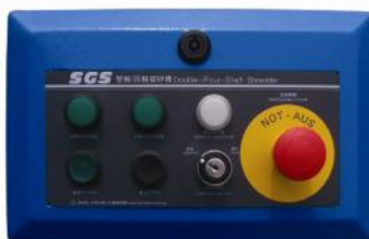
Picture 4-4: Stop / Start Button, Emergency Button
