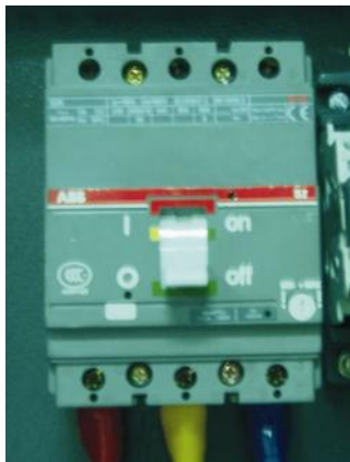
Picture 4-3: Main Power Switch
