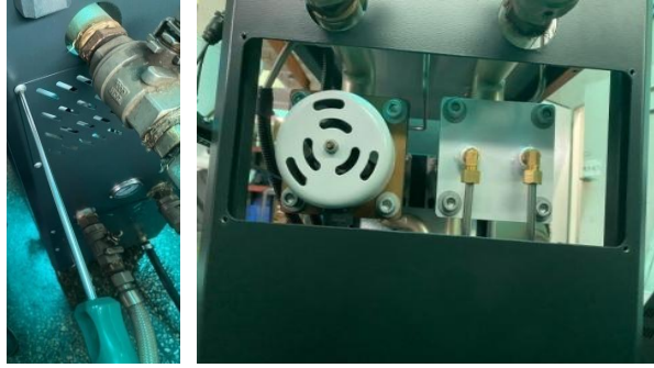
Picture 6-6: Pipe Heater 1
