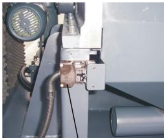
Safety switch on the storage box
