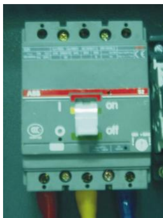
Picture 4-4: Main Power Switch
