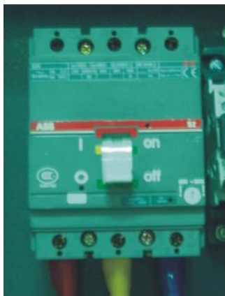
Main power switch
