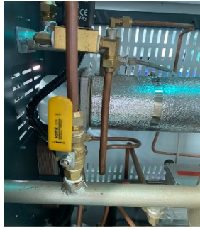
Picture 6-7: Bypass Ball Valve
