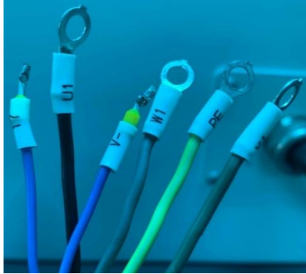
Picture 3-1-3: Blower wiring label
