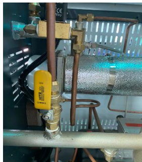
Picture 6-8: Bypass Ball Valve
