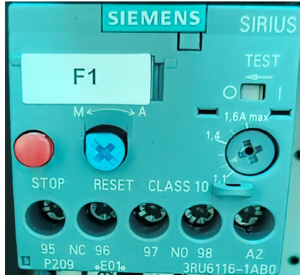
Picture 4-10: Thermal Overload Relay
