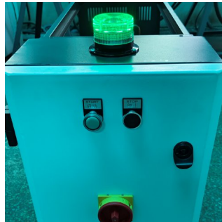
Picture 4-4: Green Alarm Light
