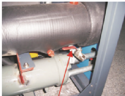
Water Drainage Port
