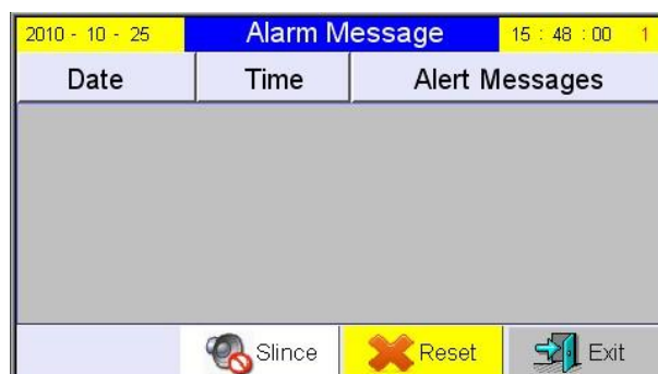
Picture 4-11: Alarm screen
