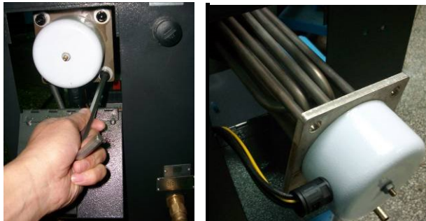
Picture 6-7: Pipe Heater 2
