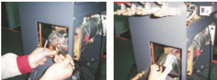
Picture 6-7: Pipe Heater 2
