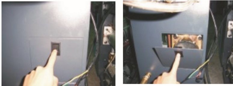
Picture 6-6: Pipe Heater 1
