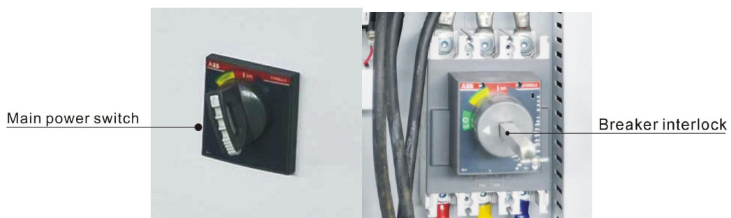
Picture 4-5: Main Power Switch
