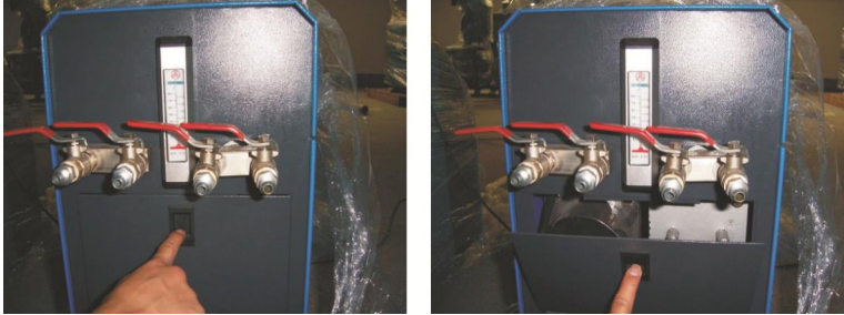
Picture 6-6: Pipe Heater 1
