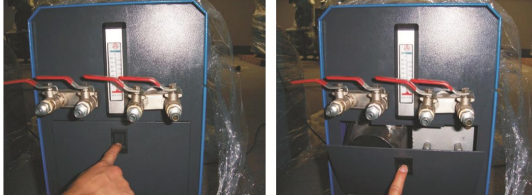
Picture 6-9: Cooling Pipes 1
