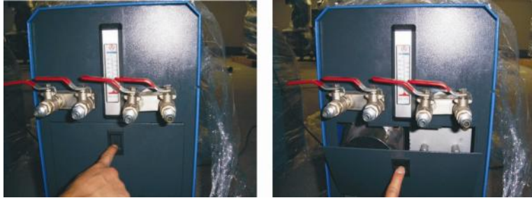
Picture 6-6: Pipe Heater 1
