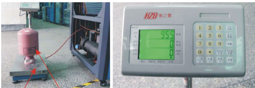
Electronic scale Refrigerant tank
