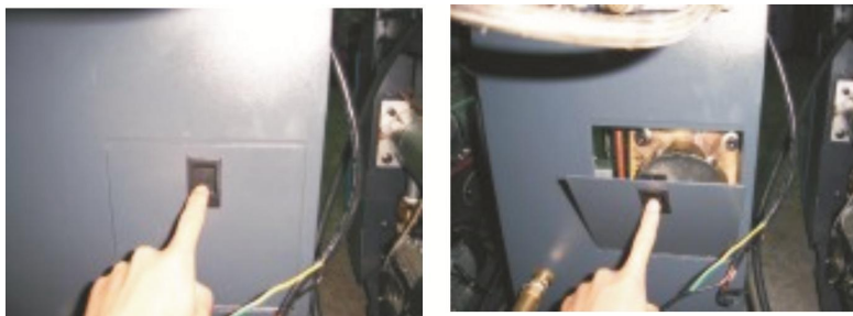
Picture 6-6: Pipe Heater 1
