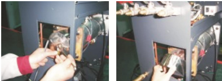
Picture 6-7: Pipe Heater 2
