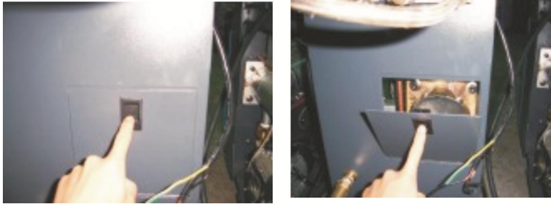
Picture 6-6: Pipe Heater 1
