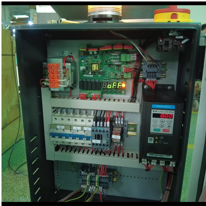
Picture 2-4: Electrical Components Description
