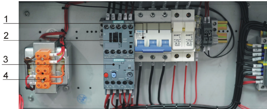
Picture 2-4: Electrical Components Description
