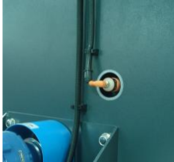
Picture 4-31: Level Switch on Mixing Tank
