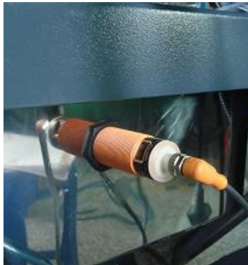
Picture 4-32: Level Switch on storage Tank
