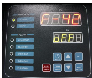
Picture 4-14: Heater Alarm
