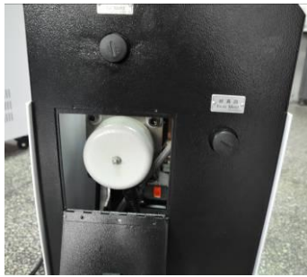
Picture 6-7: Pipe Heater 2
