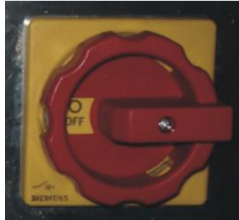
Picture 4-1: Main Switch
