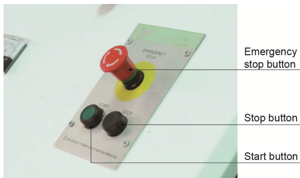
Picture 4-2: START, Emergency Button and STOP Button
