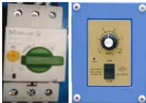
Picture 4-1 : Control Panel
