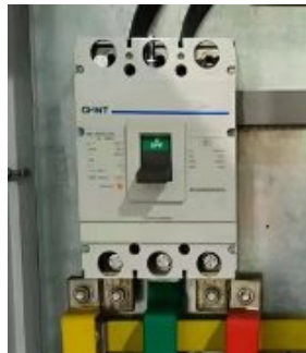
Picture 4-1: Main Power Switch
