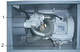
Picture 6-4: Conveying Blower
