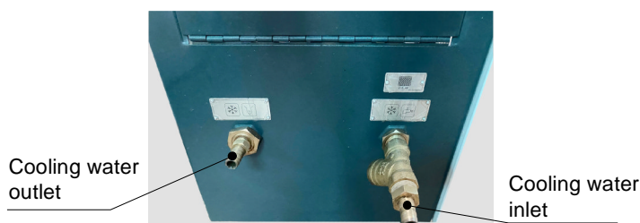
Picture 3-2: Pipe Connection
