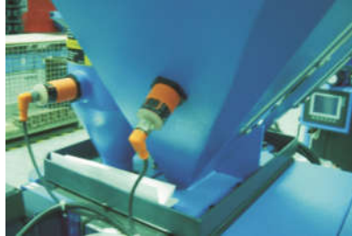
Picture 4-27: Level Switch on Hopper
