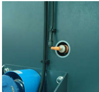
Picture 4-28: Level Switch on Mixing Tank
