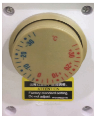
Picture 3-11: Compressor anti-freeze switch
