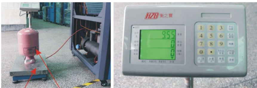
Electronic scale Refrigerant tank
