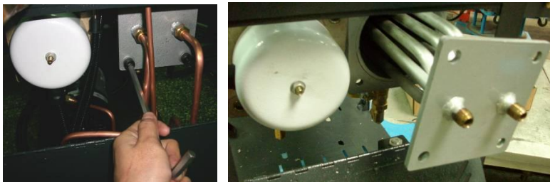
Picture 6-9: Cooling Pipes 2
