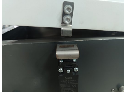
Picture 5-1: Feed box safety switch pin
